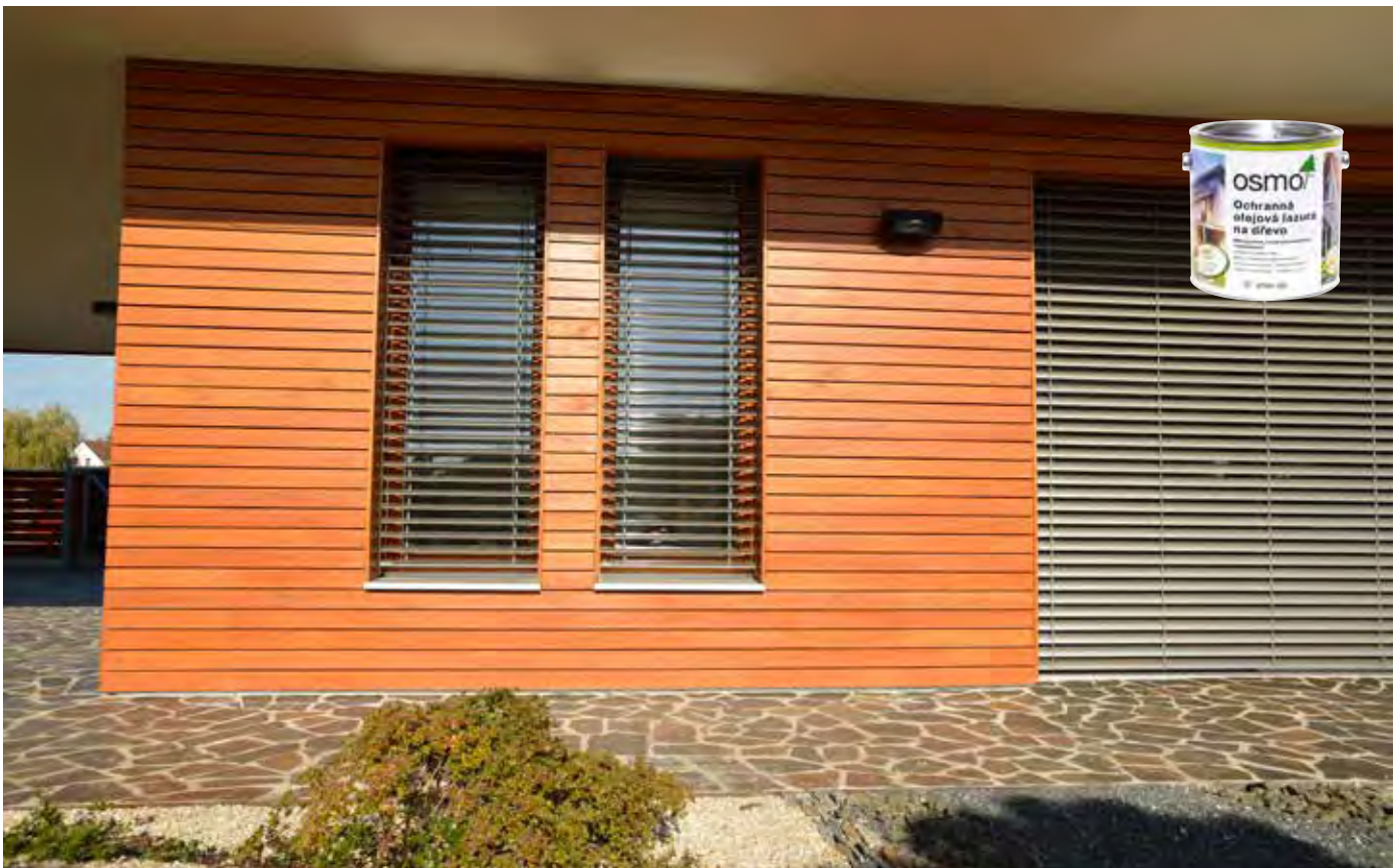
REAL FACADE, Siberian larch, Raute profile 20 x 93 mm, surface treatment OSMO Protective oil stain n. 728 Cedar
